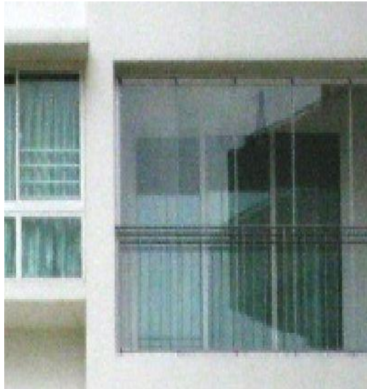
Figure 3.20 Balcony screen that is not allowed
